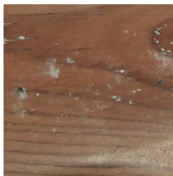
Surface mould/Mohos superficial/ Moisissures superficielles/ Oberflächlicher Moder/Muffasuperficial/ Oppervlakte-schimmel/ Bolor superficial
